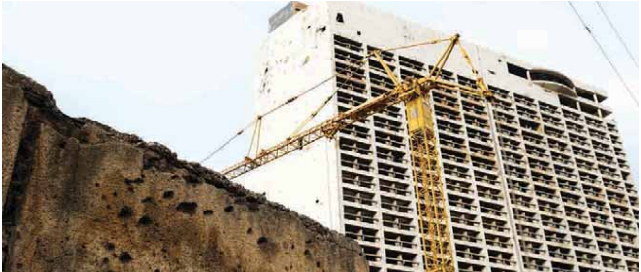
Reconstruction work in front of the bomb-scarred former Holiday Inn in Beirut, Lebanon. ©Joel Carillet/iStockPhoto
