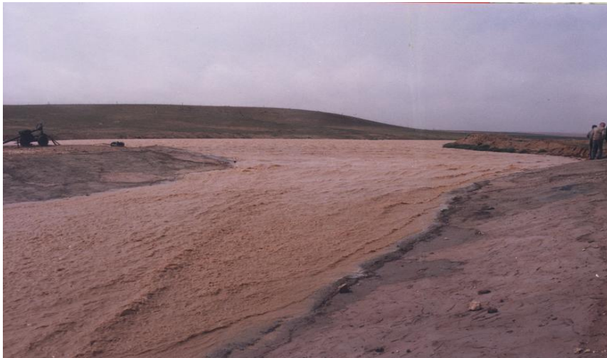
Figure 9.3: Small earth dams is used in integrated development in dry region of Jordan
