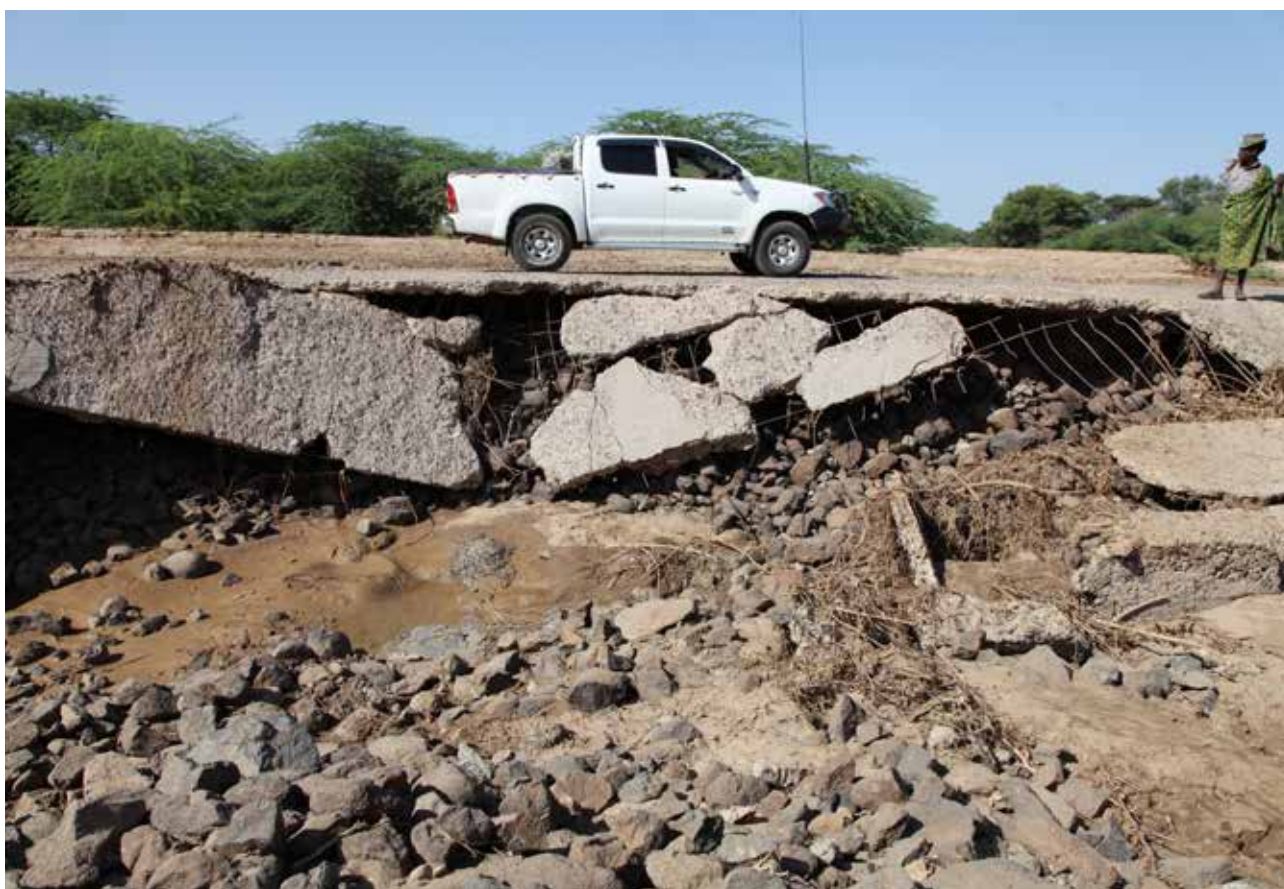
A vehicle passes by a broken bridge in Kalobeyei town in Turkana, Kenya. Photo ©UN-Habitat/Julius Mwelu.
